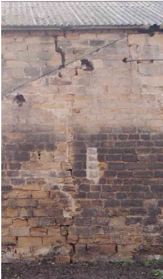
Figure 17: Barn N wall joint/crack (1995)
